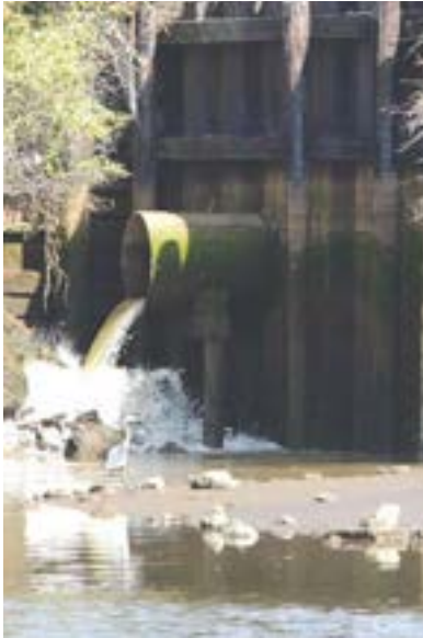
Polluted stormwater runoff continues to degrade water and sediment quality in the river
